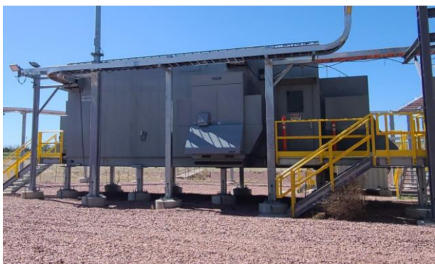
6500 HP VFD E-HOUSE
