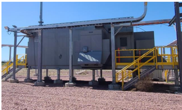
6500 HP VFD E-HOUSE
